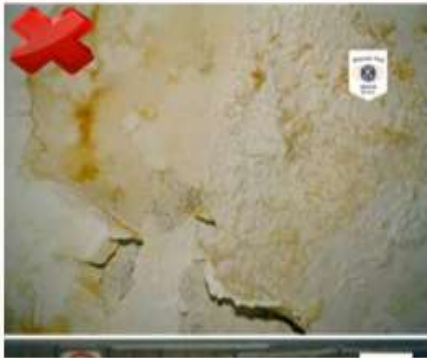
Fig.2.9 Fungal growth on the walls
