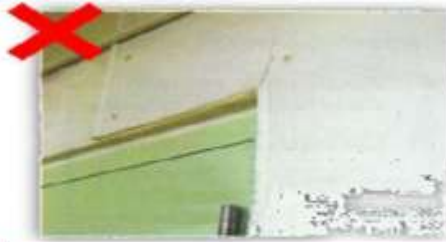
Fig.2.8 Cracks allow bacteria and moulds to accumulate.
